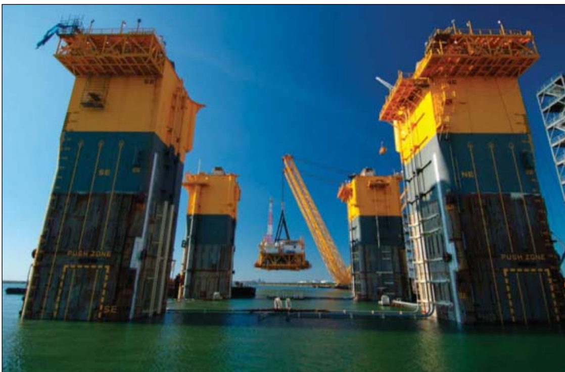
Stationary cranes lifted the topsides onto the hull on Sept. 19 (Fig. 4). Photo from Enterprise.
